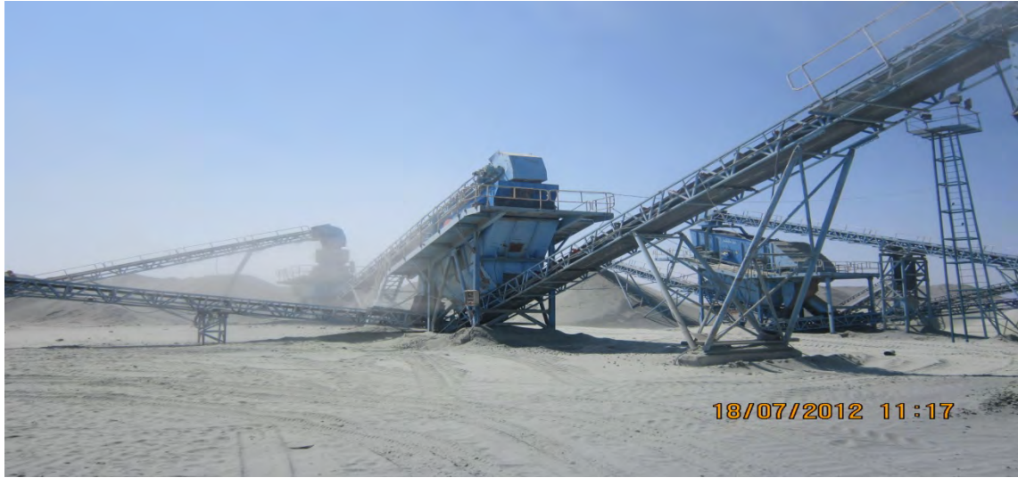
Photo 5: Stone crushing plant, Korday-By-Pass, July, 2012
