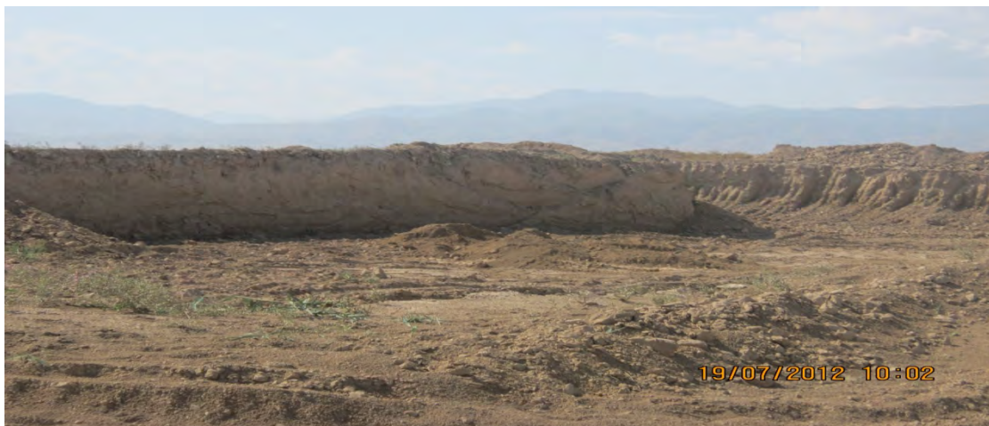
Photo 9: Excavation of borrow pits with sharp side slopes, Korday By-Pass, July, 2012
