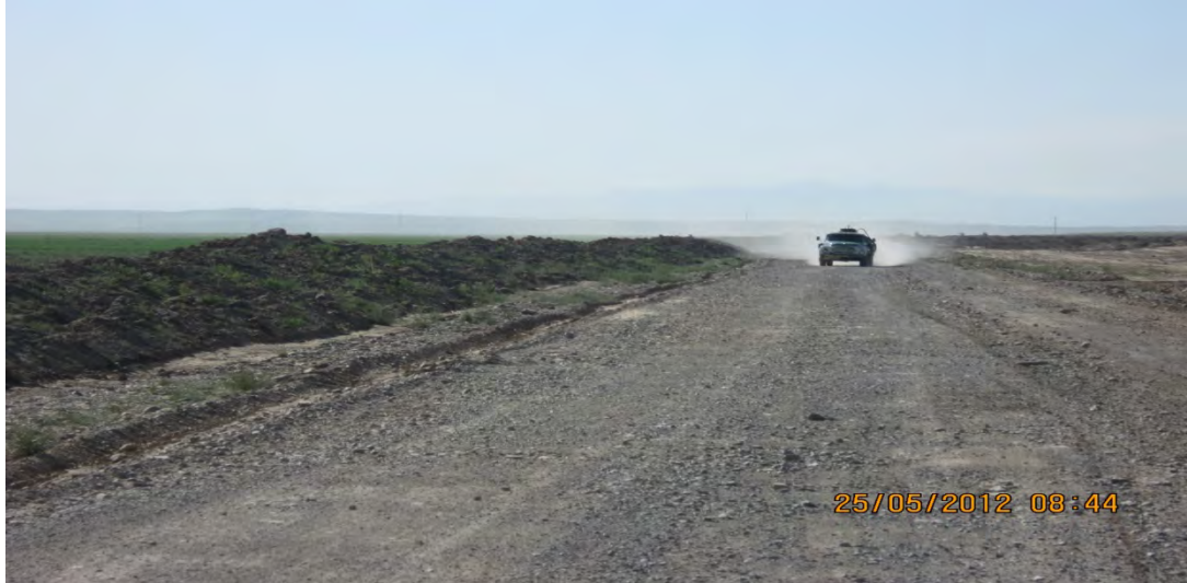
Photo 7: While carrying materials, trucks are not covered to arrest dispersion of dust, Access to Kyrgys Border, Karday, May 2012
